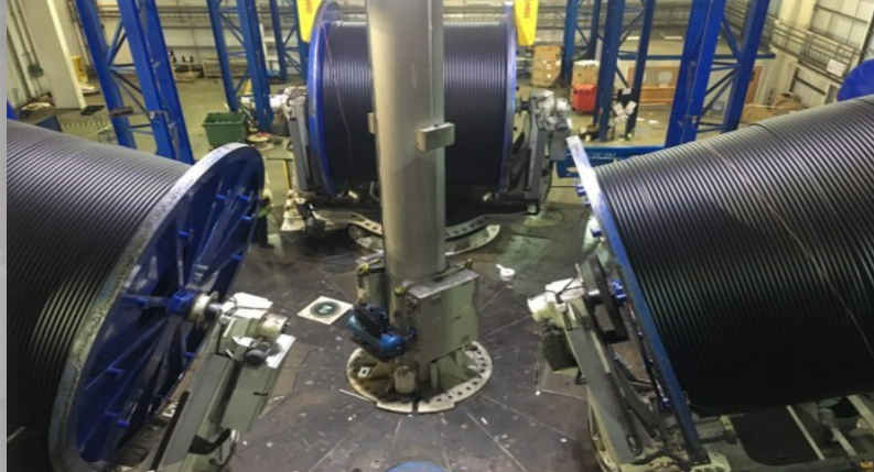
Replacement of all obsolete VSD System Installation & Commissioning of a new Centralised PLC Control System (Siemens S7-1500) & Datalogger.
